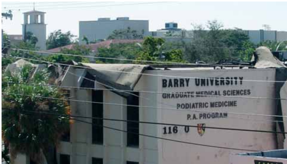
Over half million dollars damage to SGMS building
